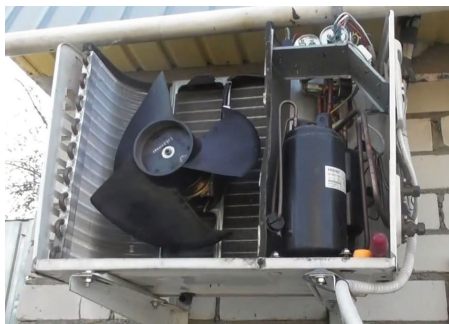
Exchanger and compressor
